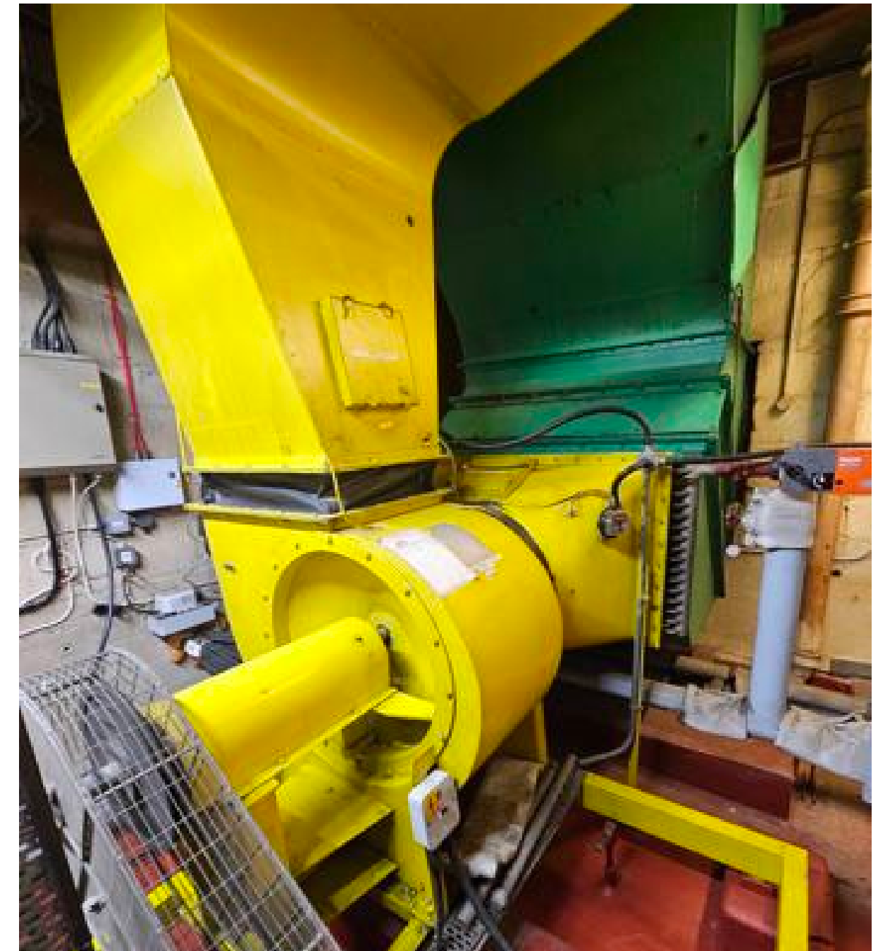
Building Ventilation Supply Fan Unit
